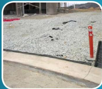
Good application of rock exit pad. Note short section of material against curb that is keeping rock from leaving site.
